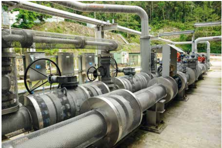
Export gas metering at the Central Processing Facility at Kutubu.
