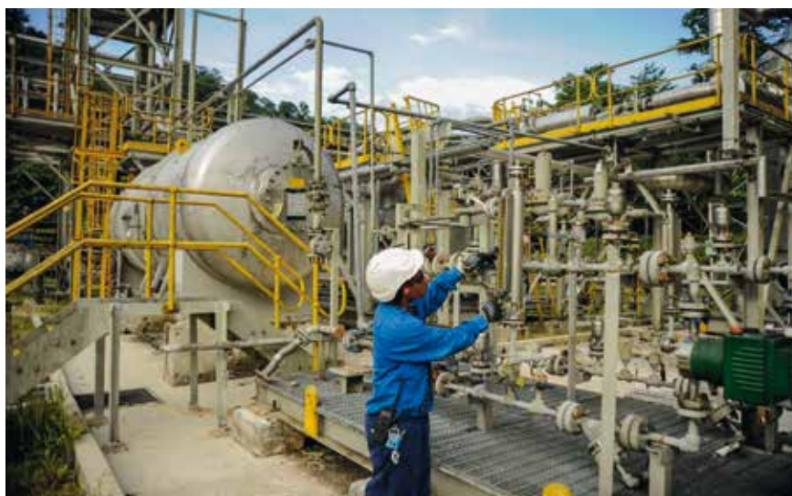
Central Processing Facility, Kutubu, PNG Highlands.
